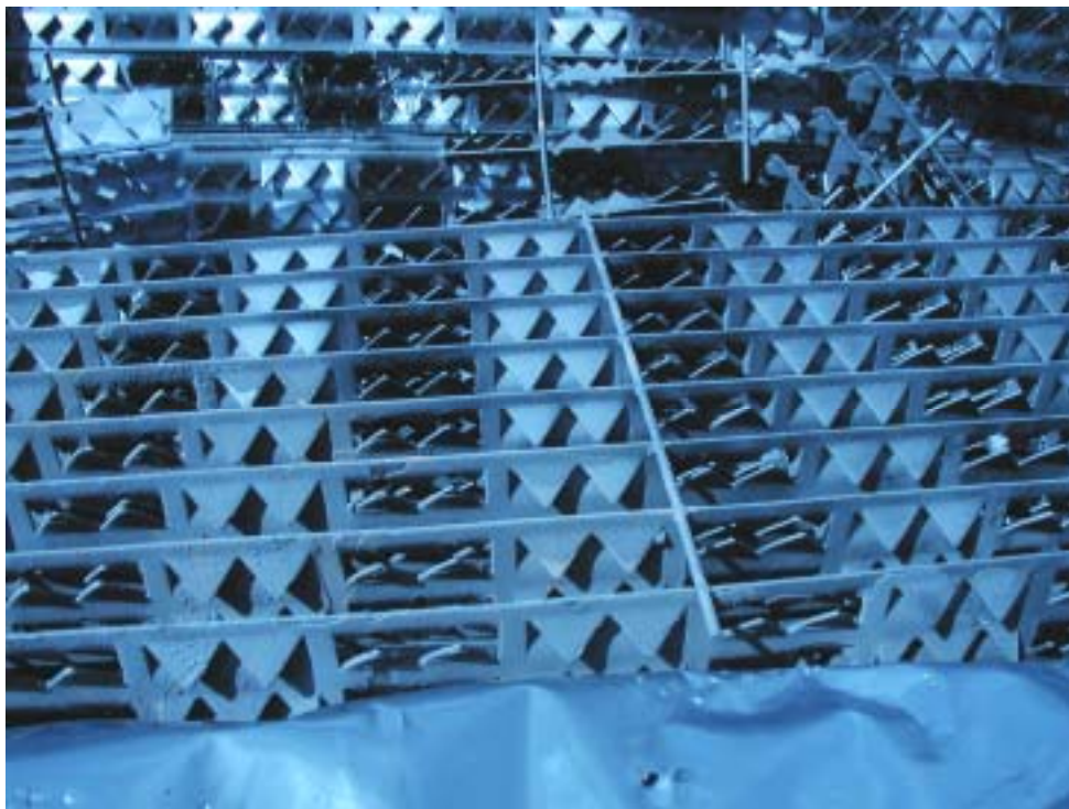
Figure 13: FLEXIGRID Style 2 Removed From Slurry Pumparound
