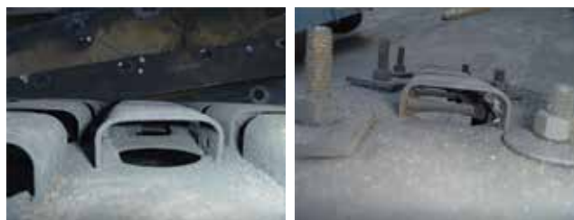
▲ Figure 16. Enhanced fixed valves had little fouling after being in service in a coker fractionator for several years.
