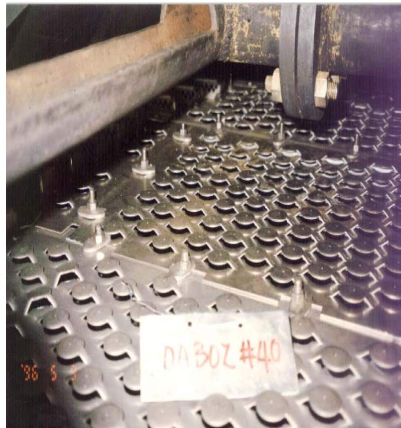
Glitsch High-Performance Anti-Fouling Tray, SUPERFLUX® "After one year in operation"
