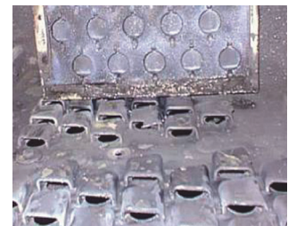
PROVALVE® orifices show little signs of fouling after 5 months.
