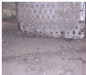
Sieve trays are more than 90% plugged after 5 months.
