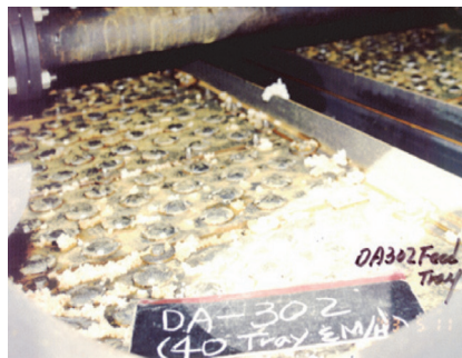
Conventional trays show severe fouling.
