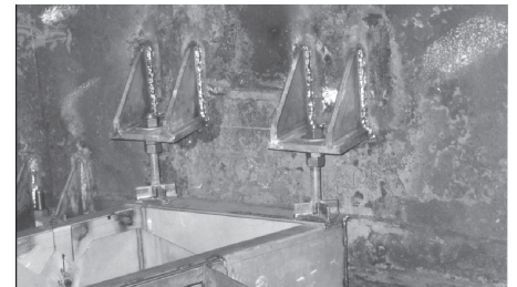
Special uplift protection design for a parting box of a liquid distributor.
