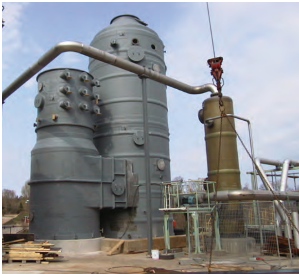
GRP Flue Gas Condensing Scrubber.
