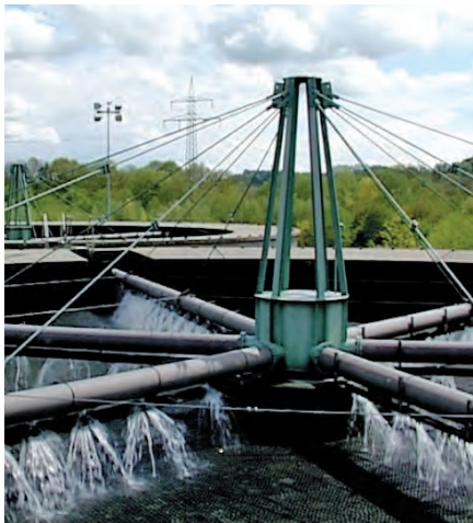
Water treatment facility.
