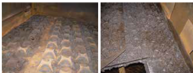
▲ Figure 15. After operating for one cycle in a coker fractionator, these moving caged valves had considerable fouling.
